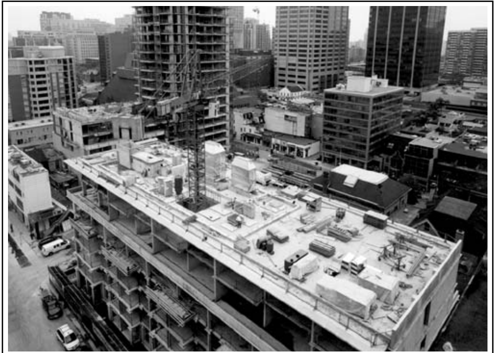
OVERLOOKING YORKVILLE □ Work progresses for the condominium project 18 Yorkville Ave. in Toronto. Construction manager Tucker Hi-Rise Construction Inc. began the 36-storey tower and seven-storey building May 2003 for owner Great Gulf Homes. There will be a total of 411 units, three levels of underground parking, a gym, media room, lounge/party room, a roof top deck and a new city park. The project was designed by architects Alliance. Consultants are: Yolles Partnership (structural); The ECE Group Ltd. (mechanical/electrical); and Janet Rosenberg & Associates (landscape). Subtrades include: Anpro Excavating & Grading Ltd.; Deep Foundations Contractors Inc. (shoring); Resform Construction Ltd. (formwork); Gilbert Steel (rebar supply); Innocon Inc. (concrete supply); D. Zentil Mechanical Ltd.; Nortown Electrical Contractors Associates; and ThyssenKrupp Elevator Ltd.
